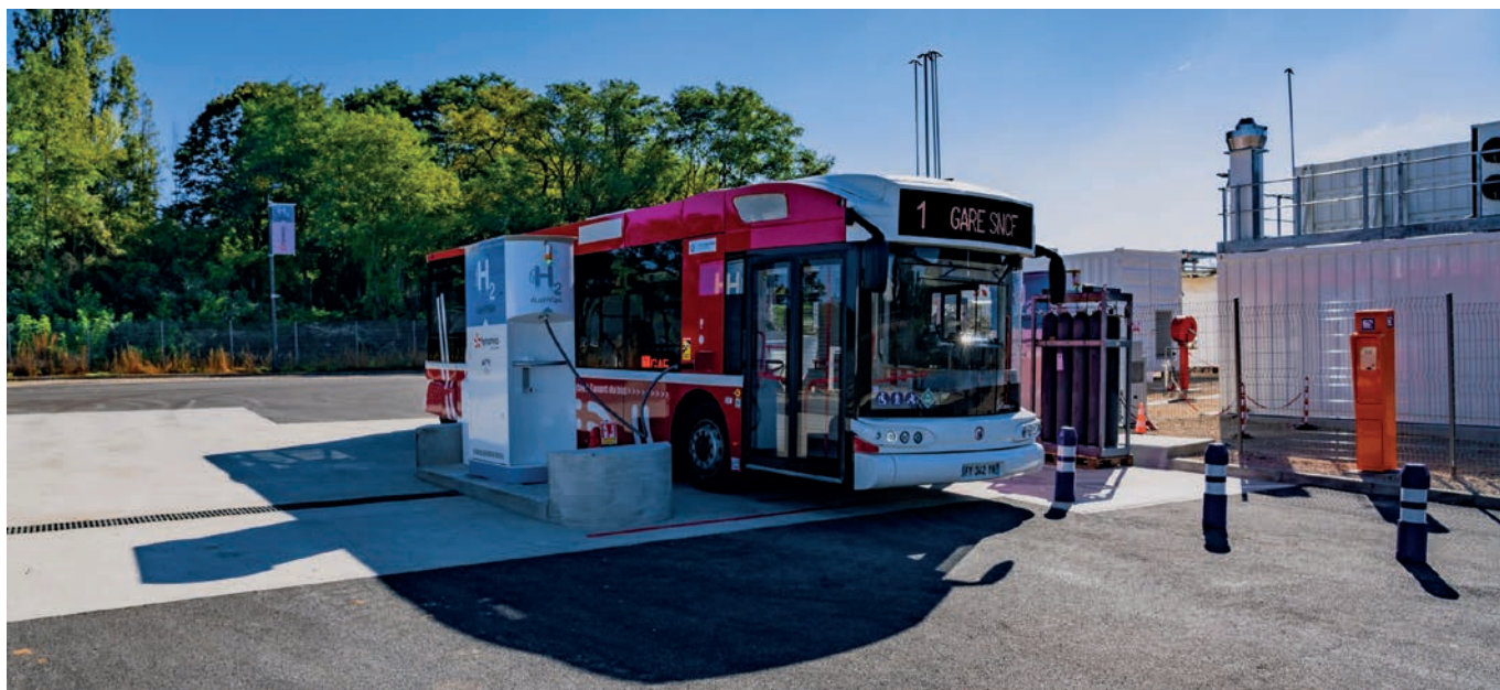
AuxHYGen project: Low-carbon hydrogen stations for buses in France (400 kg of hydrogen per day, 1 MW electrolysis capacity) to supply 5 buses.
